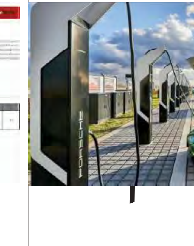
J CHARGING STATION (AC) 2 Public Accessible located on Haynes Street
