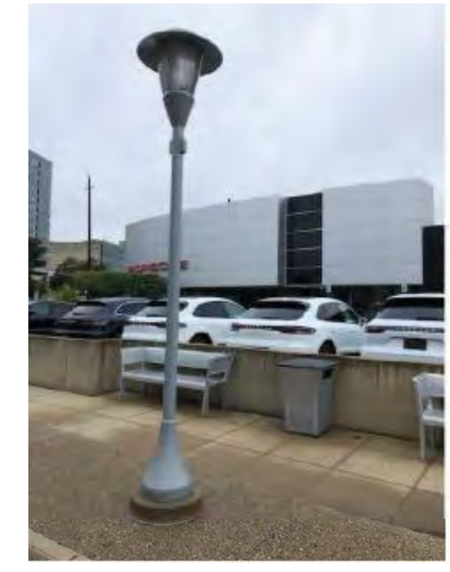
E EXISTING + NEW STREETLIGHTS (BLX + SL-F) Luminaire Street Light Model P190-42-W To conform with Triangle District Standards
